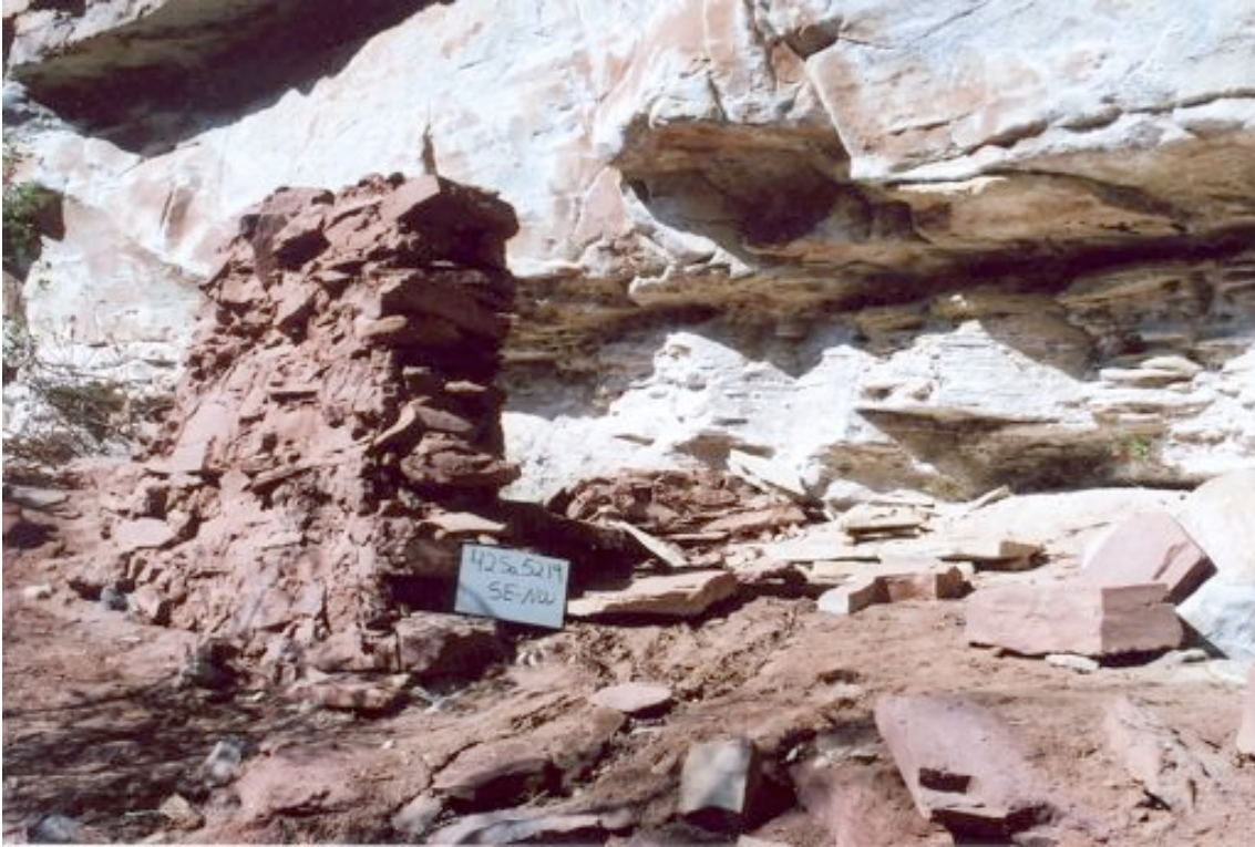
Figure 13: Severe erosion at 42Sa5219 has impacted the structural integrity and could expose subsurface cultural materials.
